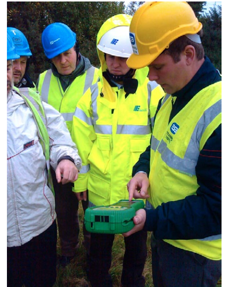
2. Measurement of ground resistance.
